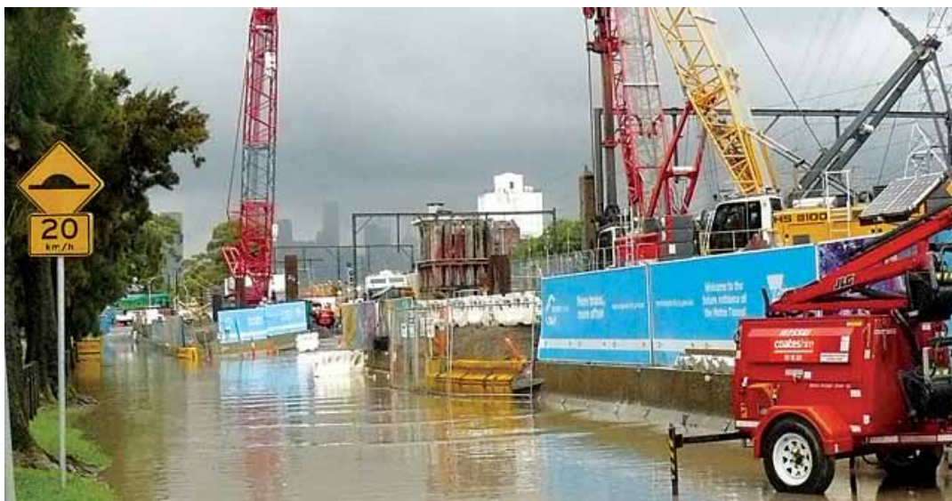
Work goes on at the Metro Tunnel entrance in South Kensington despite the rain. Photograph: Janet Graham
